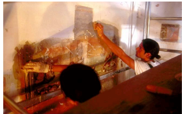
Figure 1. A traditional approach to art diagnosis and restoration In this example, a sample region was scraped to determine what lay beneath the wall paint (see the patch on the right side of the image). At one depth, the diagnosticians found a fresco, and the restorers chose to uncover the entire wall to that layer.
